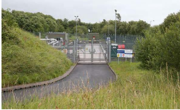
Image 2.1 Typical Pressure Reduction Station
