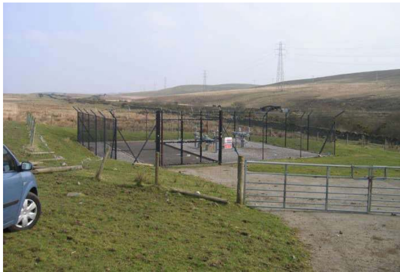
Image 2.2 Typical Block Valve
